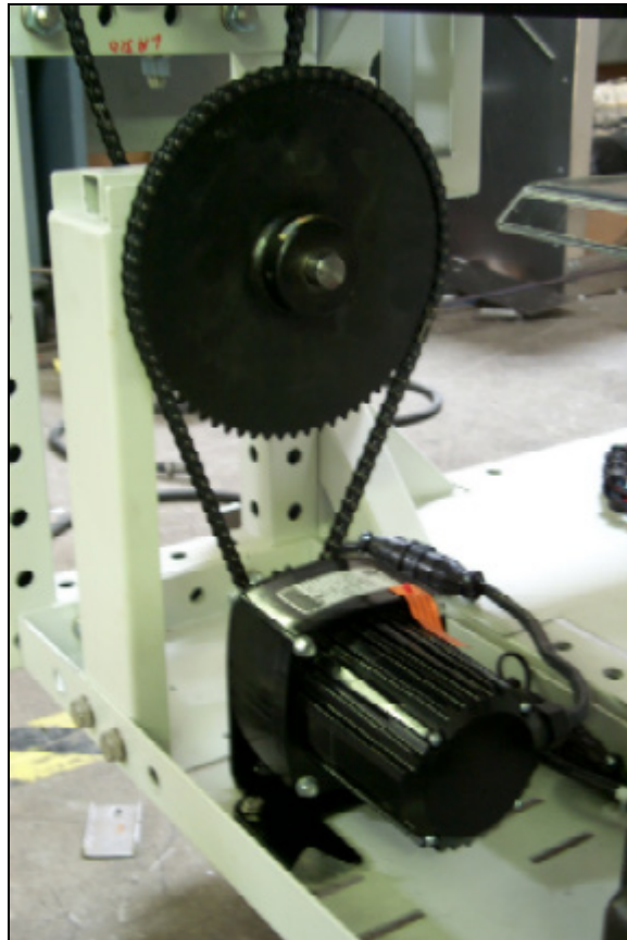
Figure 3-7: Conveyor Belt Motor
