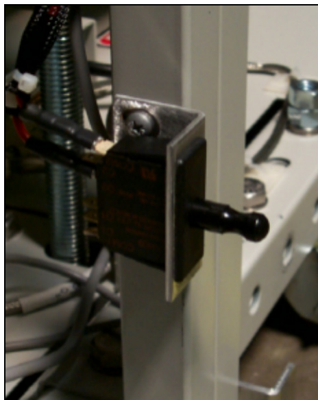
Figure 2-2: Panel Switch Installed (Override Mode Position)
