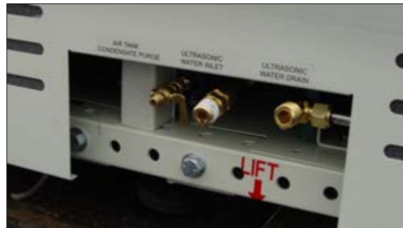
Figure 2-31 UCD Water Connections with Air Purge
