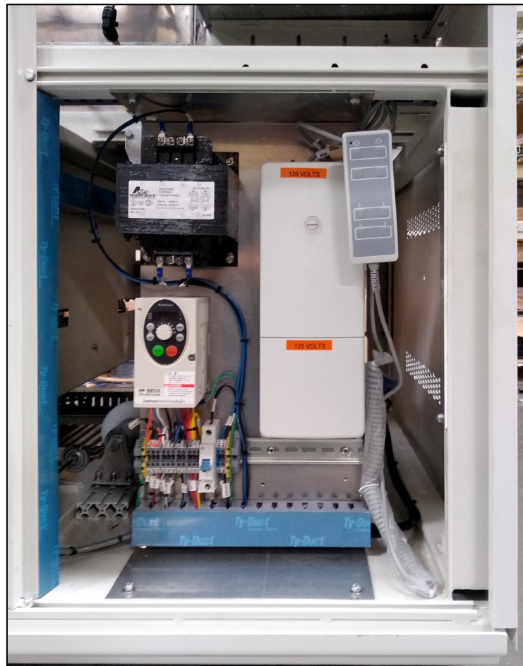
Figure 4-14 MCL Controller at Front Exit
