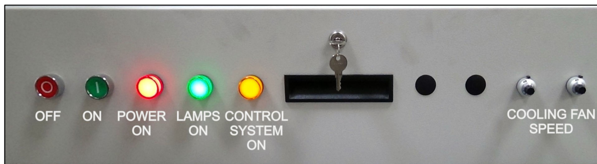
Figure 3-2 Control Console Furnace Power ON and OFF & Indicator Lights
