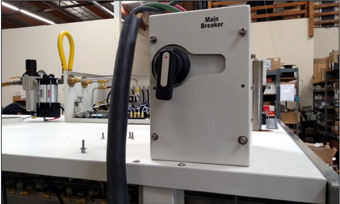
Figure 2-20 Top mount circuit breaker
