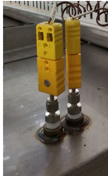
Figure 1-43 Redundant Type K Thermocouples
