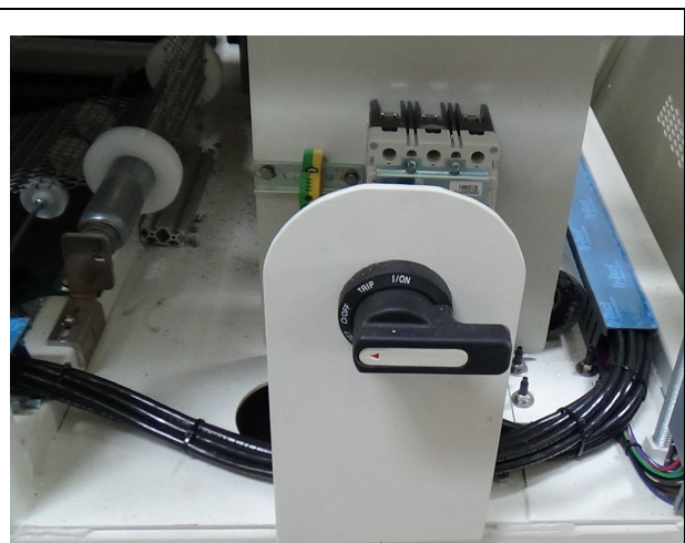
Figure1-24 3-Phase Circuit Breaker-Panel OFF
