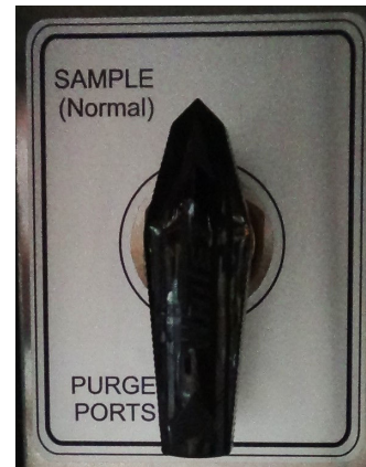
Figure 4-23 Sample–Purge valve on OSS panel
