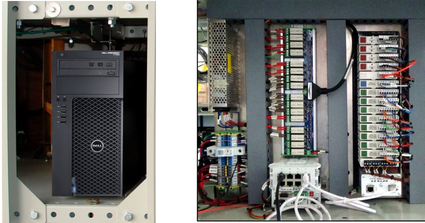
Figure 4-17 Computer and UPS (L) PLC panel (R)
