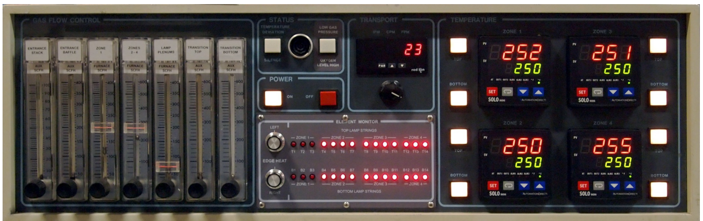
Figure 3-1 Furnace Control Console
