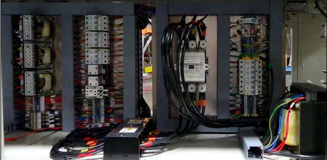
Figure 3-12 Power Distribution and Safety panels
