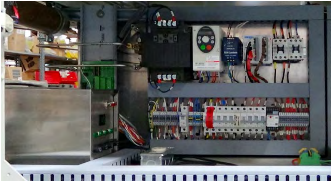
Figure 3-13 MCC / UCD panel
