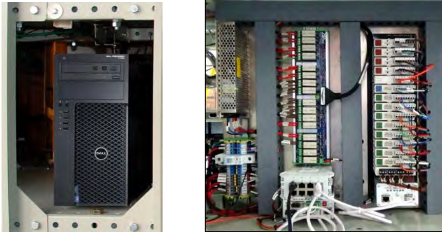
Figure 3-15 Computer and UPS (L) PLC panel (R)
