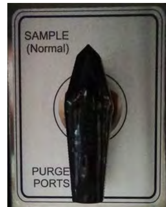
Figure 3-21 Sample–Purge valve on OSS panel
