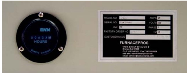
Figure 1-17 Elapsed Time Meter and Nameplate
