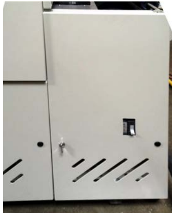
Figure 1-19 Circuit Breaker panel
