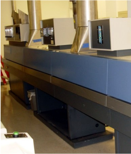
Figure 1-33 Cabinet Exhaust Example
