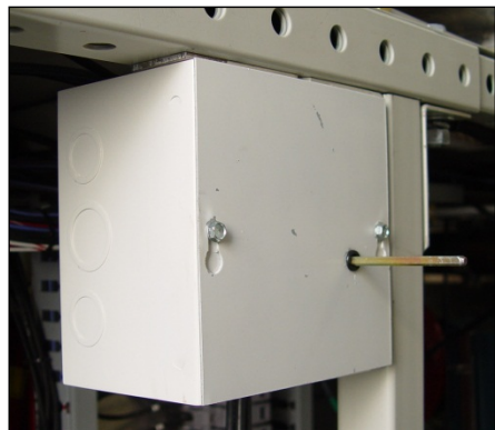
Figure 1-21 Interlock disconnect switch enclosure
