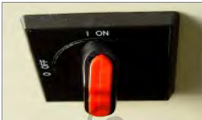
Figure 2-9 FURNACE Interlocked ON/OFF switch
