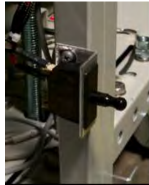
Panel Switch Installed - Bypass Mode Position
