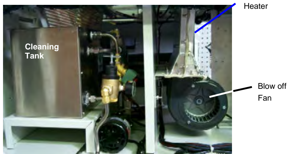
Figure 0-17 Ultrasonic Cleaner installation
